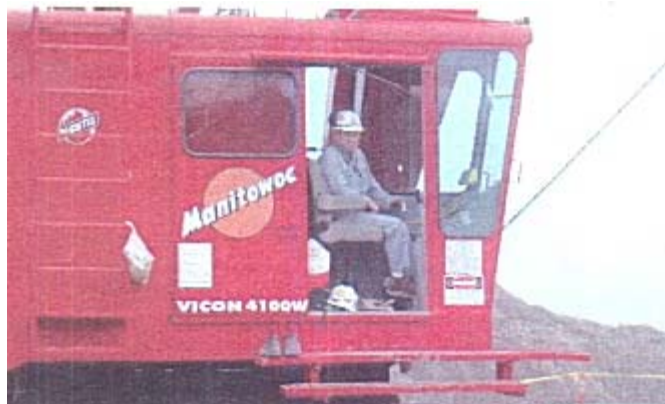
Above, Russell Retzack in a 230 ton capacity crane at the Oak Creek power plant job site, January 2006
